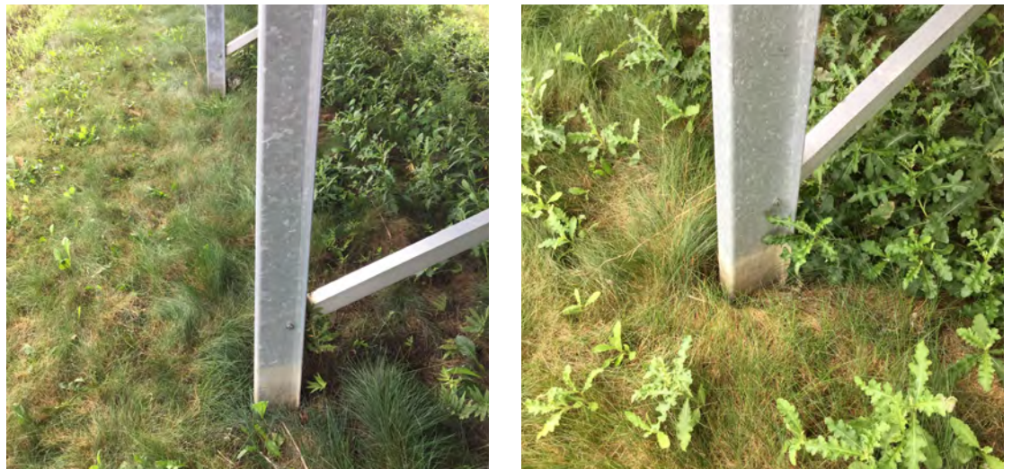
Figure 6: Frost heave effect on piles
