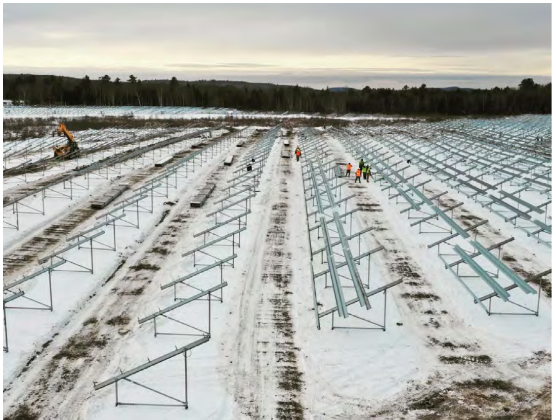
Figure 12: Utility solar project in Milo, Maine utilizing GLIDE Agile
